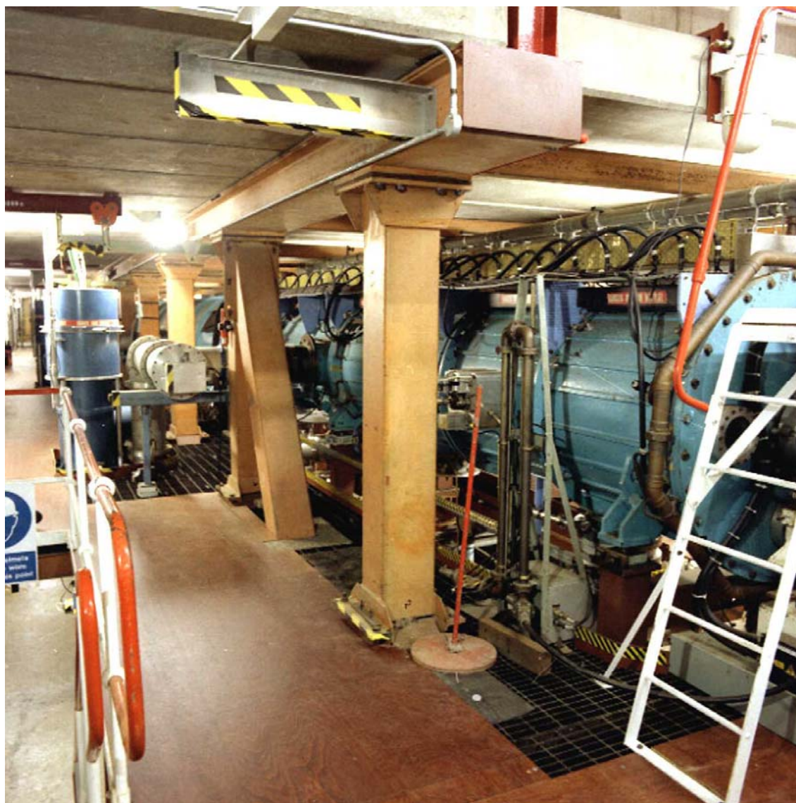
View down north side of ISIS 70 MeV H - linac
