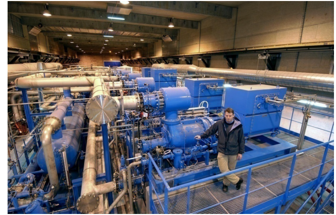
CERN cryogenic plant
