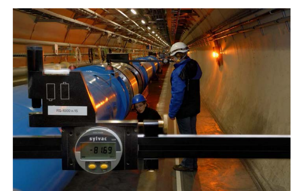
Wire offset measurements in the LHC tunnel
