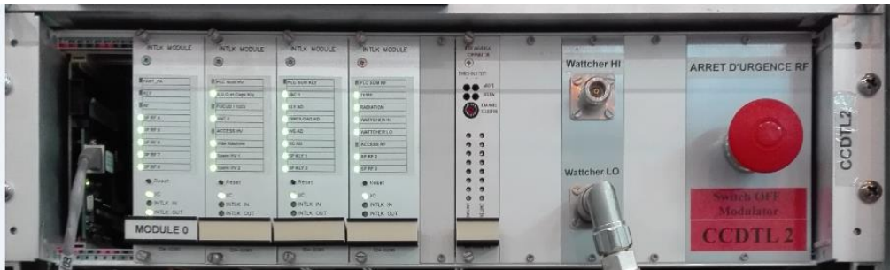
An example of interlock system for LINAC 4
