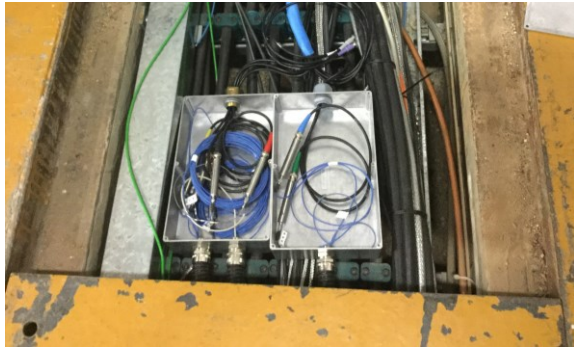
Figure 3 – Termination boxes housing in-line conditioning amplifiers and wiring beneath synchrotron hall floor
