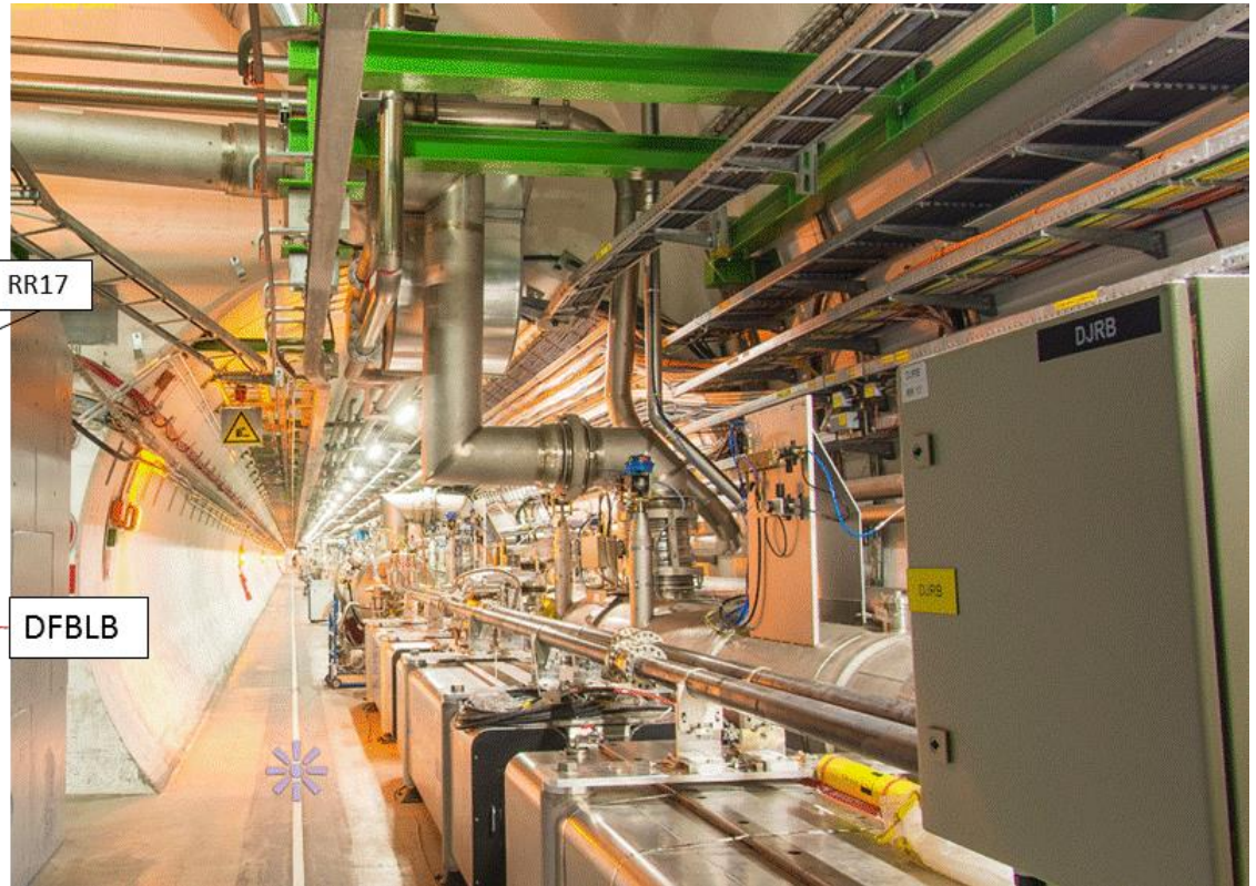
DSL in LHC tunnel
