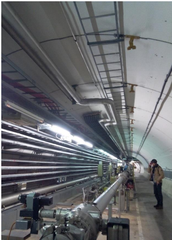
Figure 1 The U on the two raw water pipes at the tunnel vault is on top of the future crab cavity zone.
