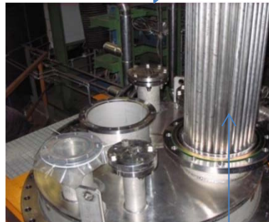
Lead-water, double-wall bayonet-tube bundle heat exchanger at Brasimone site.
