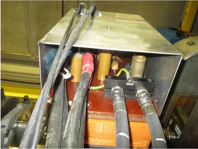
Example of non compliant cover Source: PS-CSAP 34th Meeting
