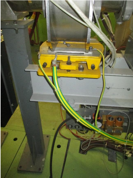
Electrical ground not connected Source: PS-CSAP 34th Meeting
