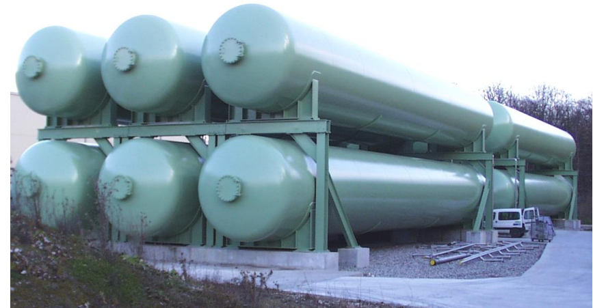
2 MPa gas tanks
