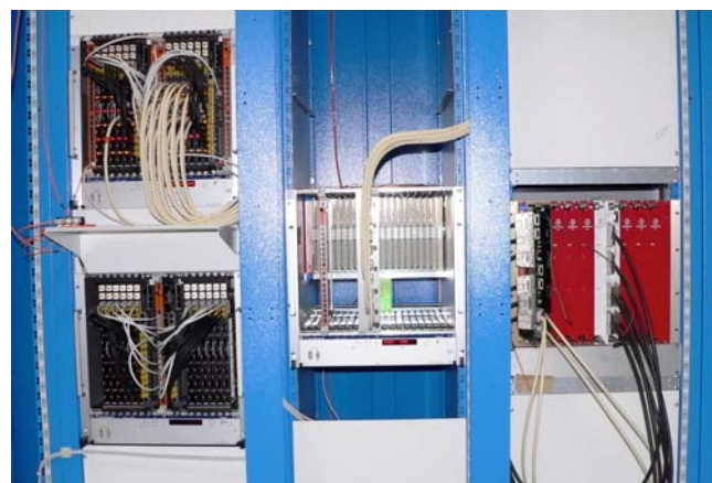
Figure 4: Front of the HCAL (right), ECAL (center), and RCT (left) racks at the integration facility. The top crate of the HCAL has the 19 cables attached to SLBs mounted on HTR cards. The ECAL rack has the TCC with SLBs and cables. The RCT has 6 cables (black) from the JSC to the JCC, and two cables (beige) from the CCC to the JCC.
