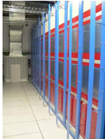
Figure 8: RCT Racks underground with crates and infrastructure. No boards have been installed yet.
