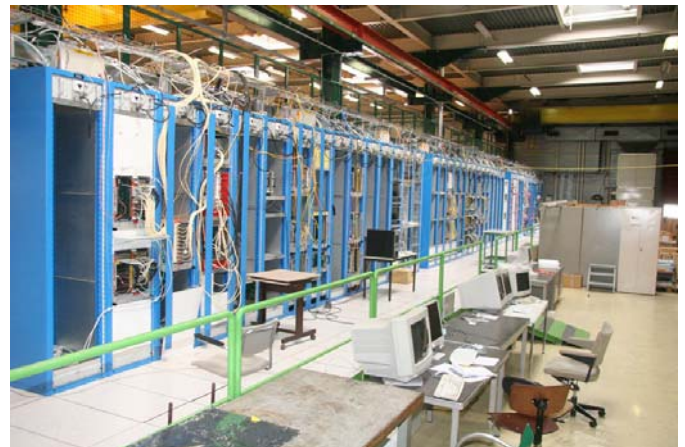
Figure 2: The integration area in the CMS Electronics Integration Centre; the first 15 racks are for system integration, the second 15 are for burn-in, and the last 15 are being used for burn-in of the low voltage power supplies.
