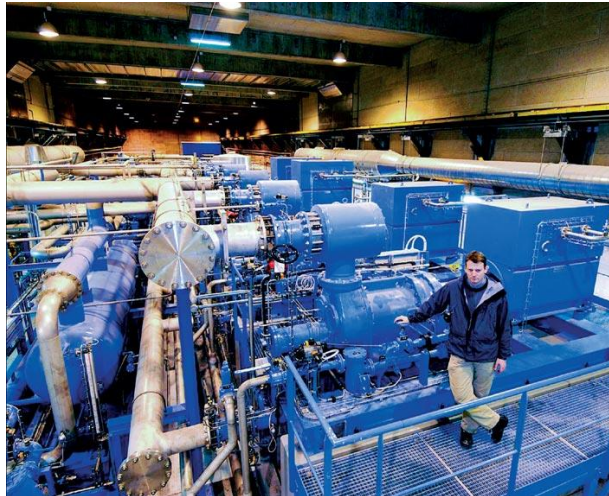
LHC warm compressor station
