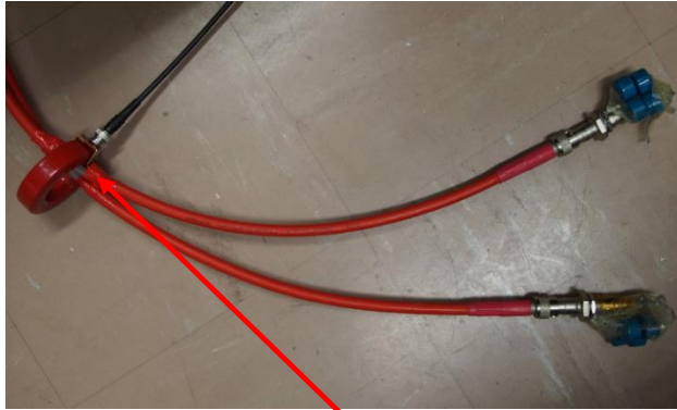
A single current transformer to measure 2 pulses, with opposite polarities.
