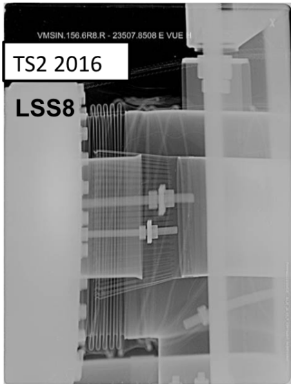
Figure 8: LSS8 vacuum module shows that a missing spring has caused rf fingers to no longer be in contact. This can cause heating due to the excitation of resonant modes with frequencies close to the beam spectrum.
