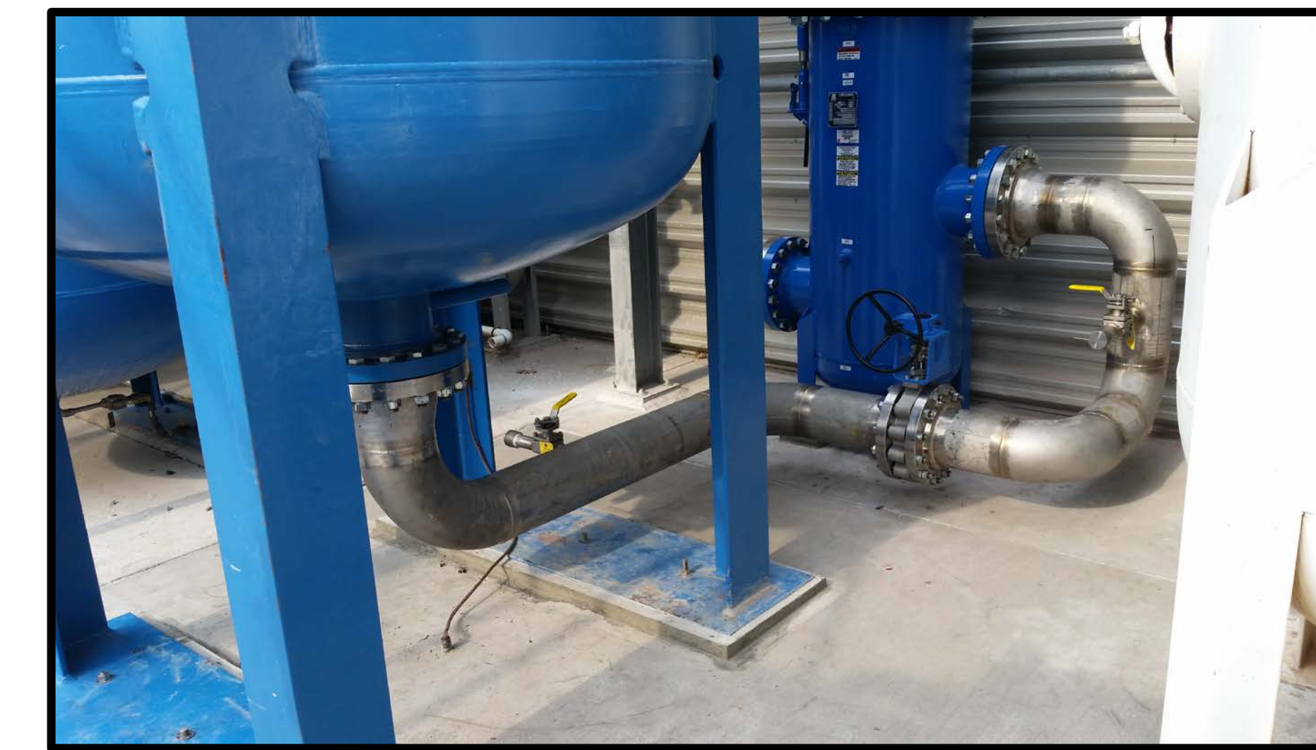
Installed Final Filter with Connecting Piping
