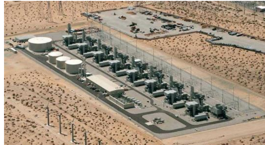
CPV Sentinel Energy Project, image courtesy of GE Energy Financial Services
