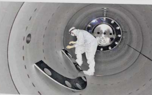
A worker installed a baffle in 2010 to control light in the Laser Interferometer Gravitational-Wave Observatory in Hanford, Wash.
