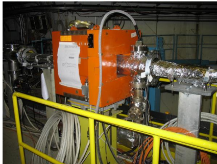
Installed in MDHW BA5 SPS
