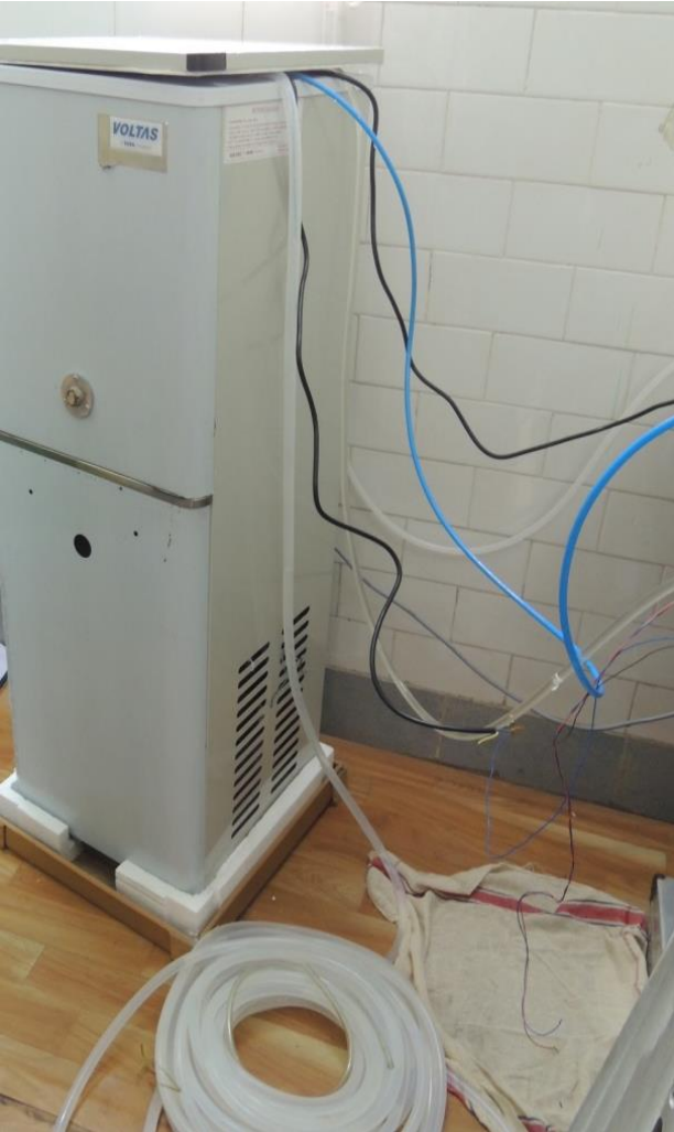
Water Chiller (sink)
