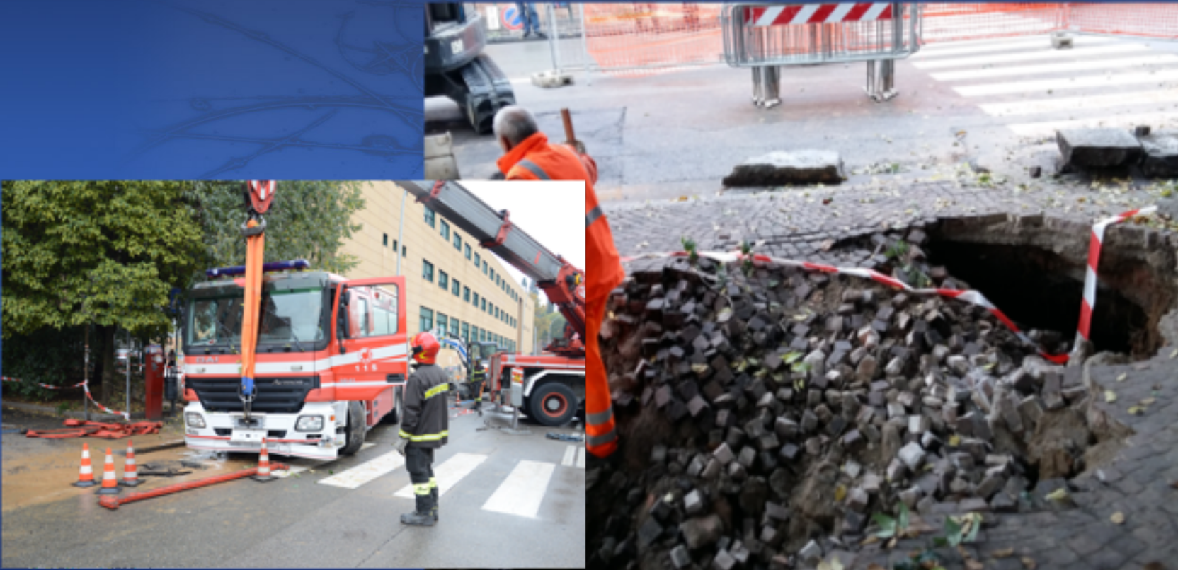
The road collapsed under the weight of the fire truck at CNAF entrance
