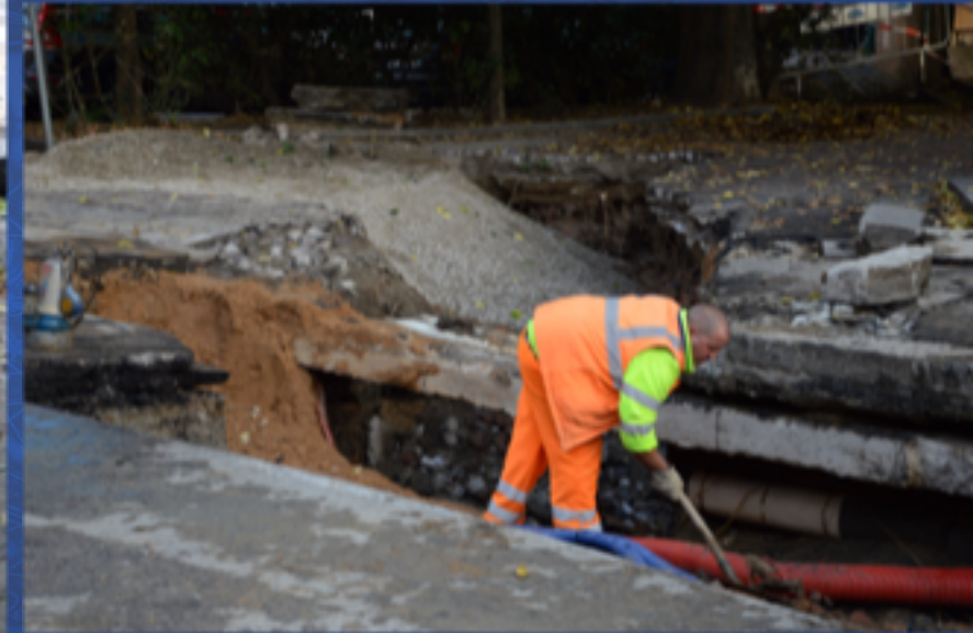
Men at work on broken pipe
