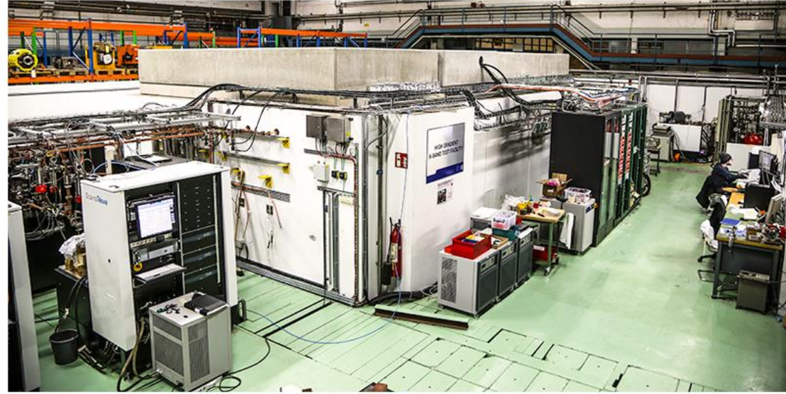
The high-gradient X-band test facility (left-side view) at CERN (Image: Matteo Volpi)
