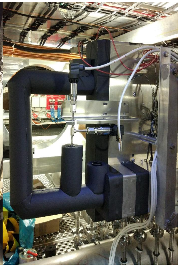
New By-pass in Manifold box
