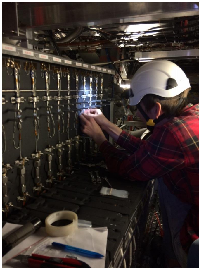
Gaskets with orifice installation
