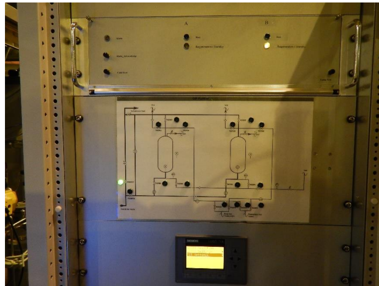
Monitoring and controls panel
