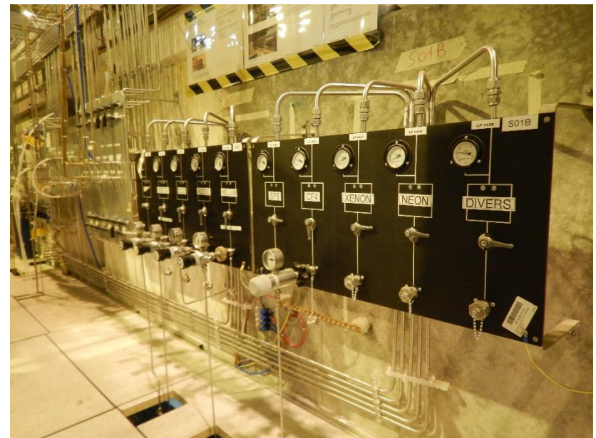
Example of neutral gas supply panels
