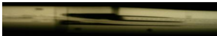
Cross-section of the interconnection and radiography showing missing continuity [F. Bordry, J. P. Tock and LS1 team]
