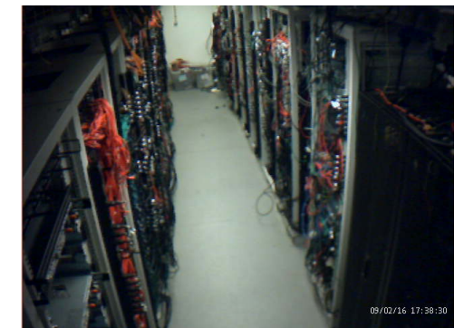
SRIF room hot aisle
