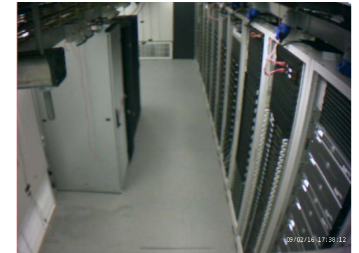
SRIF room cold aisle row 1/2
