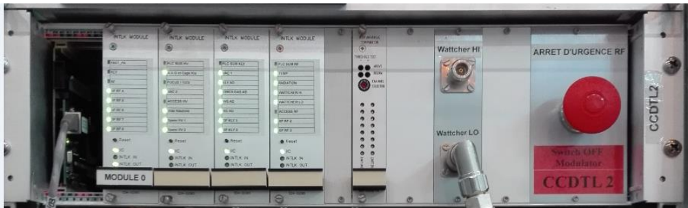
An example of interlock system for LINAC 4
