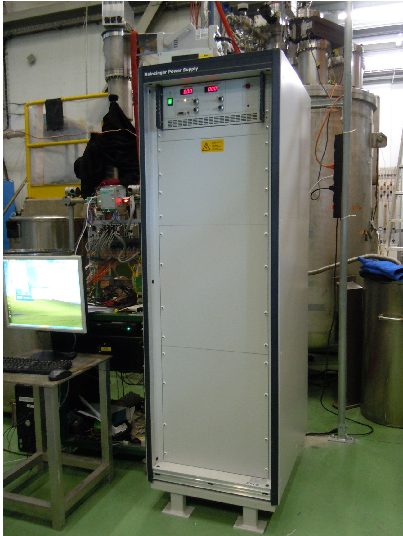
Heinzinger 300 kV Power supply
