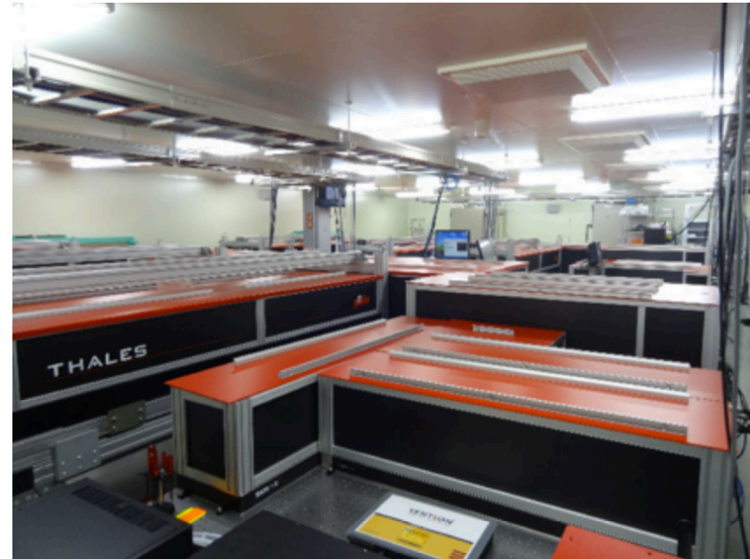
THALES PW Lase (under installation)
