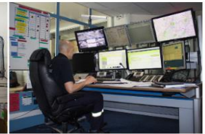
The Fire Brigade's Safety Control Room, which receives level 3 alarms.
