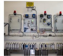
The test platform for detecting gas (including ODH). The bottles at the bottom of the image contain different types of gas used for tests.
