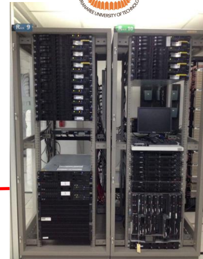
ALICE resource at Data Center
