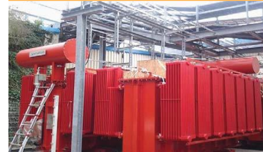
New transformers of dipole PC
