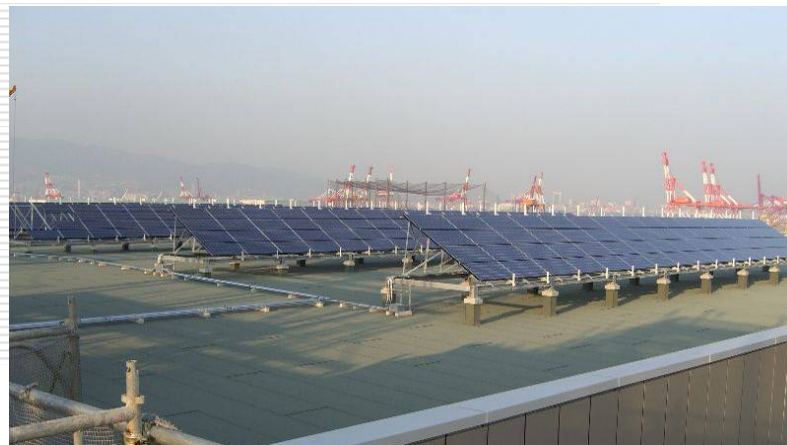
Solar panels on the top
