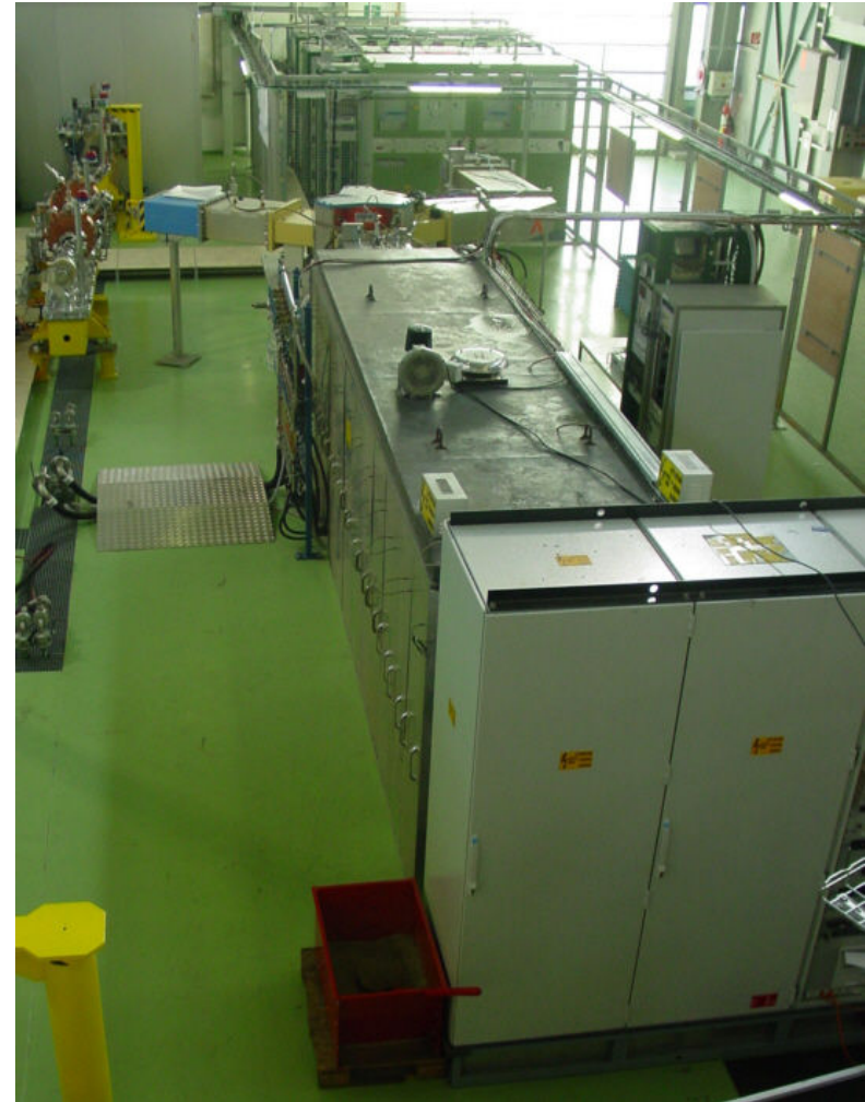
LEP-type klystron and prototype modulator under test
