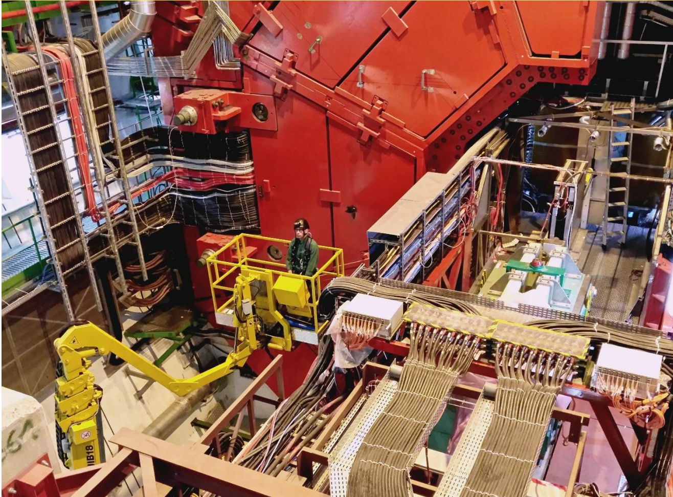
L3 magnet control and cooling systems maintenance
