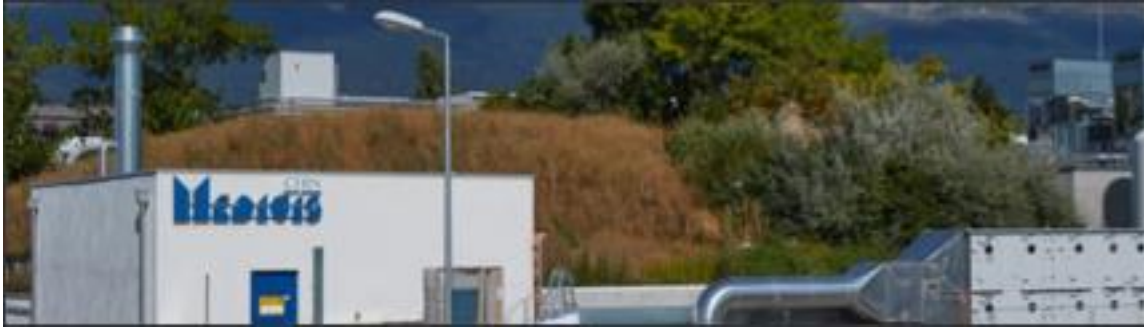
Ventilation and cooling
