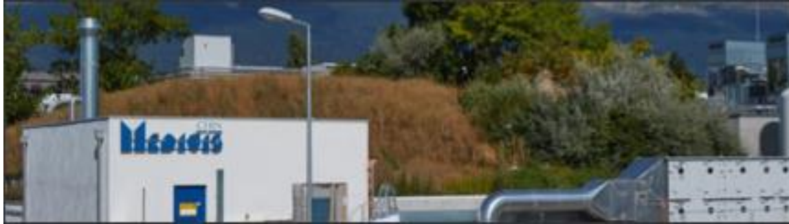
Ventilation and cooling
