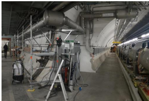
Cryogenic distribution line
