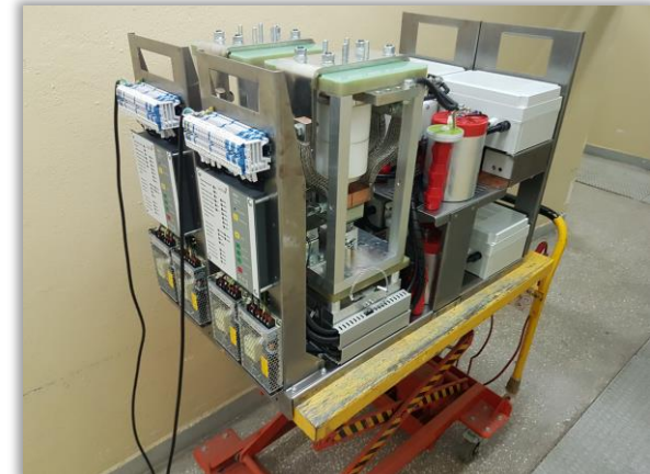
Two vacuum switches built in a sliding cassettes
