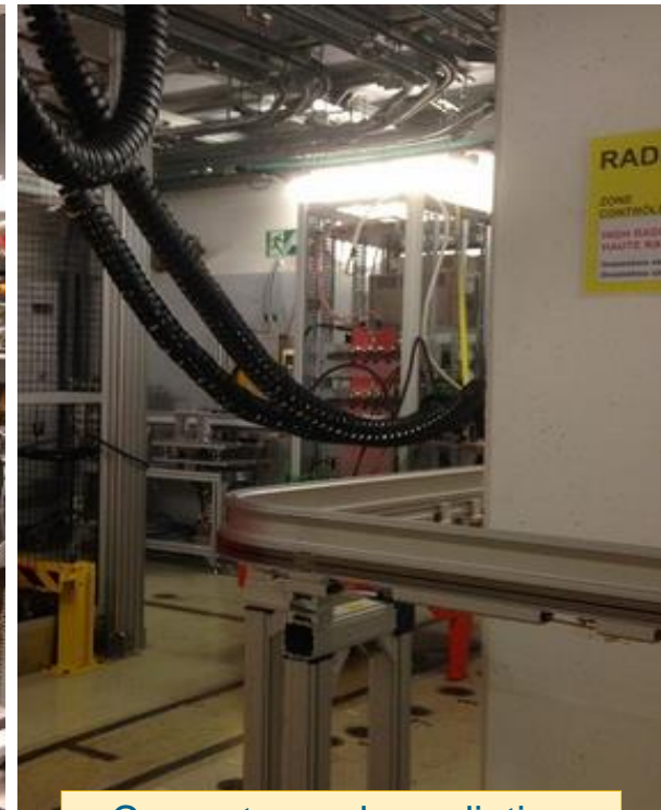
Converter under radiation
