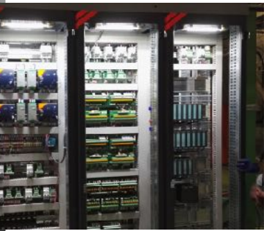
cryogenic installation (piping+ monitoring)
