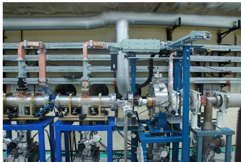
Waveguide system connected to the PWT linac.
