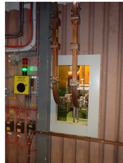
Waveguides from building 2001 to 2010
