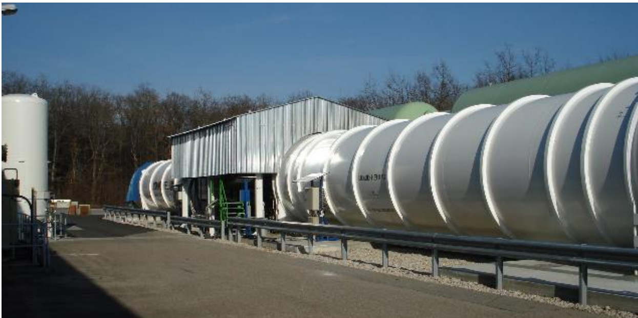
Two LHC LHe storage tanks at Point 18
