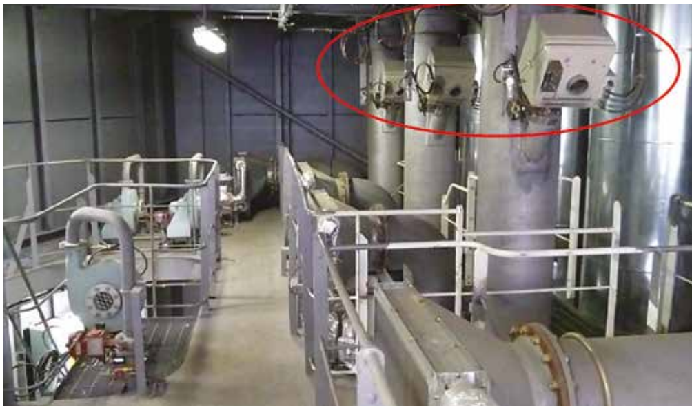
Figure 20: Continuous emissions monitoring systems (Image courtesy of Hamworthy-Krystallon)
