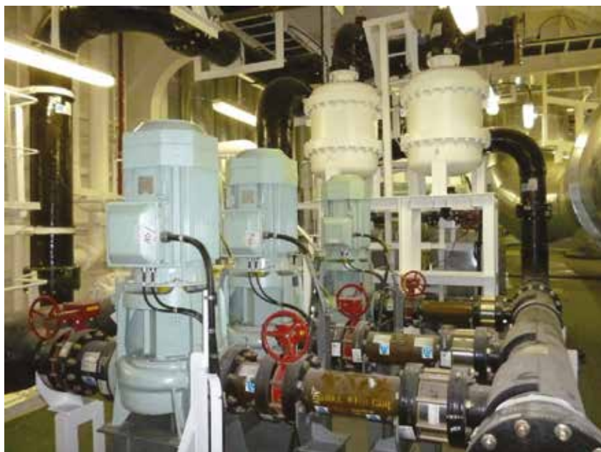
Figure 10: Washwater treatment system with GRE piping (image courtesy of Hamworthy-Krystallon)
