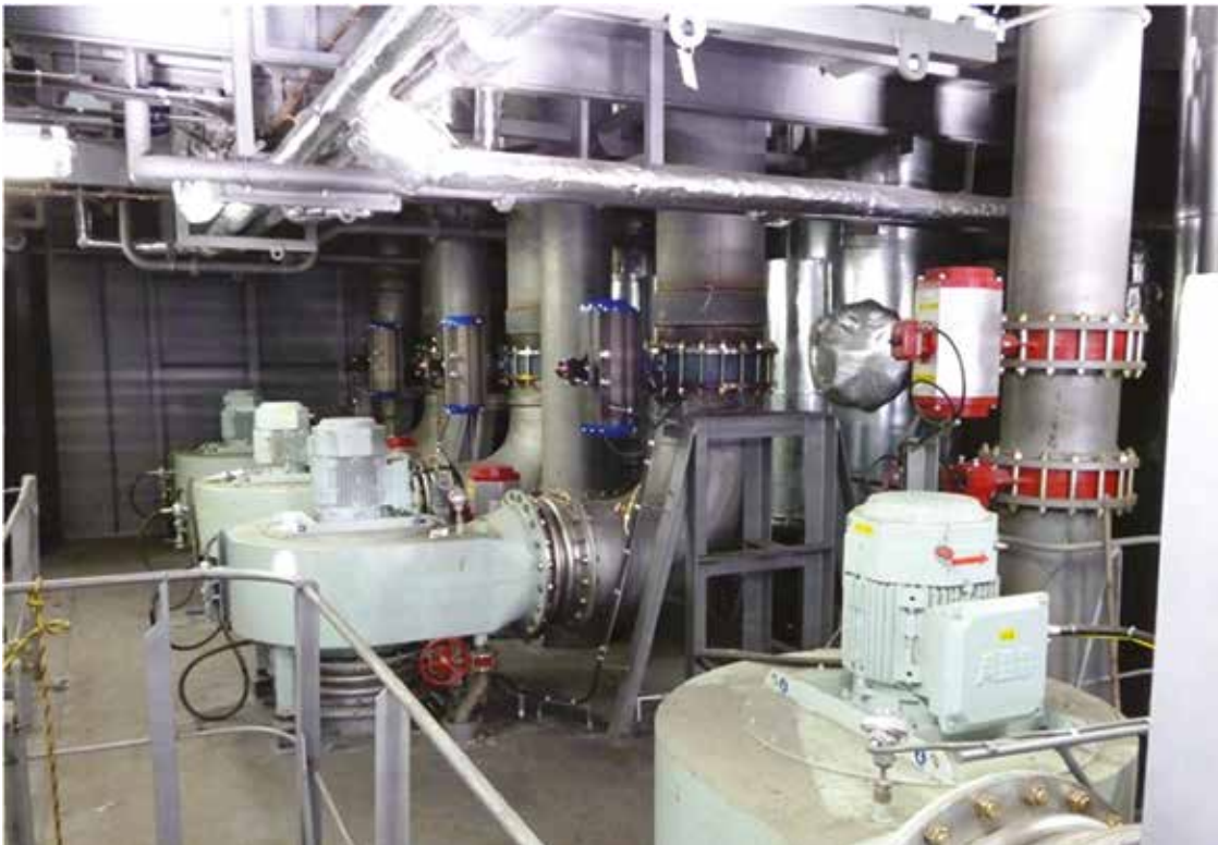
Figure 18: ID fans in exhaust ducts (image courtesy of Hamworthy-Krystallon)
