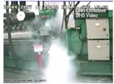
Department of Homeland Security video shows a generator spewing smoke after a staged experiment.
