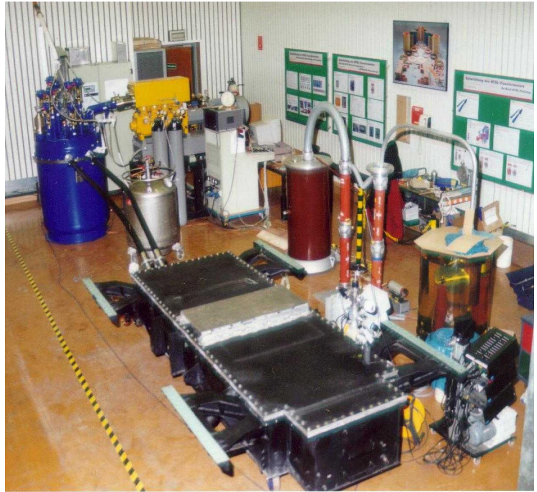
HTS-Transformer in test field
