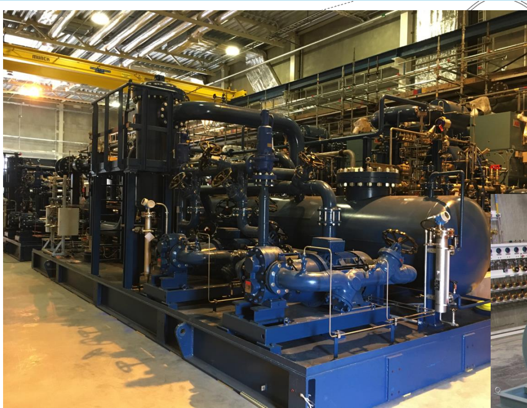
ACCP compressors and oil removal system
