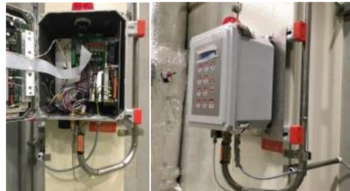
Oxygen Deficiency Hazard system
