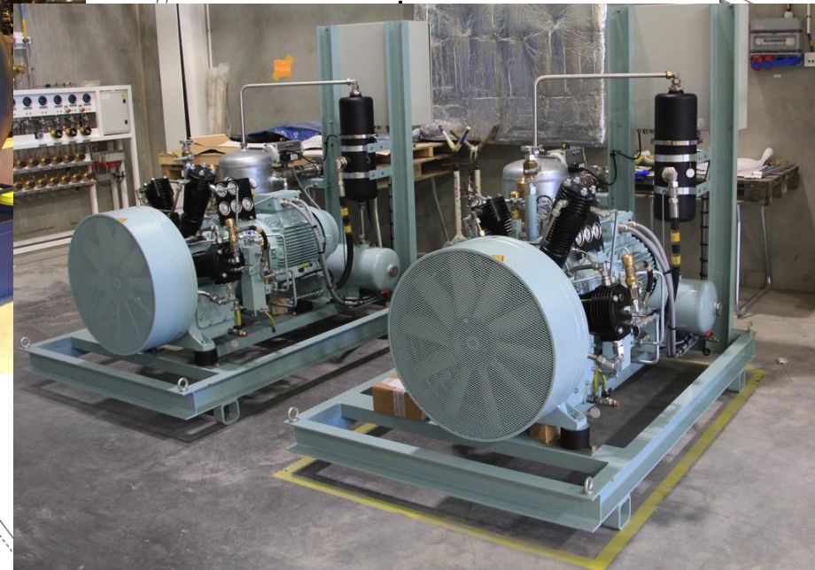
Helium Recovery System Compressors
