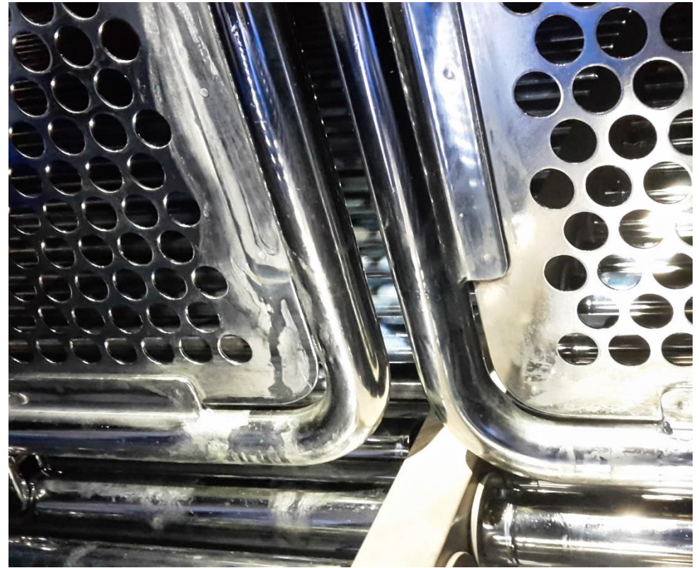
Vessel #1 - Dry stains on the panels
